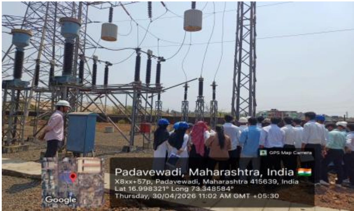
MSETCL Officer elaborating the substation infrastructures to the students
