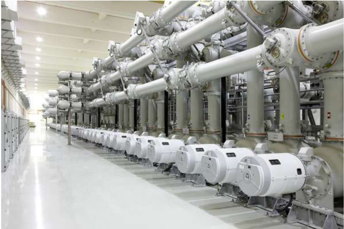
400KV Gas Insulated Substation (C.P)
